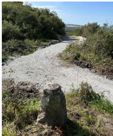
Photograph 1: The new pathway alongside Trelavour. A bench, dog waste bins and new gates have been installed.
