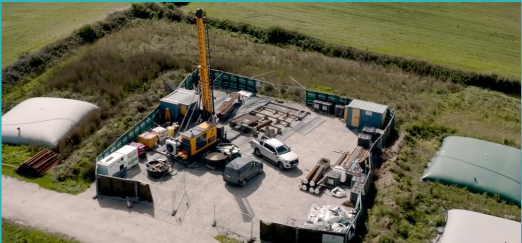
An aerial image of a similar exploration drill site at Cross Lanes, near Chacewater. The drill rig mast extends to 12 metres and fits on a standard lorry.
